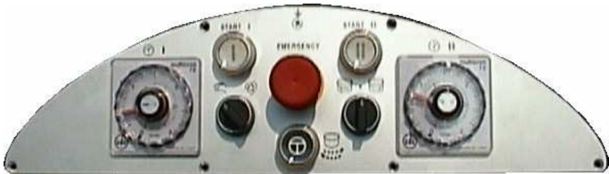
Fig. 5.1: Control panel CPM
